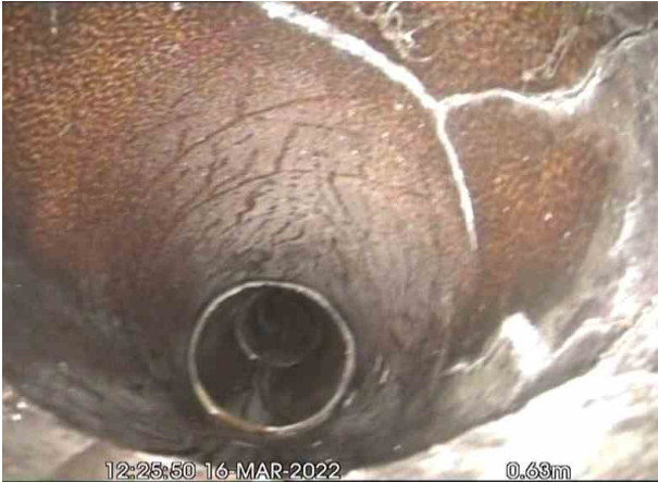
MH6X_5309bed7-a537-438a-8c0b-1f0c109ae0b2_20220325_153220_137.jpg, 00:00:05, 0.63 m Fracture, circumferential from 10 o'clock to 2 o'clock
