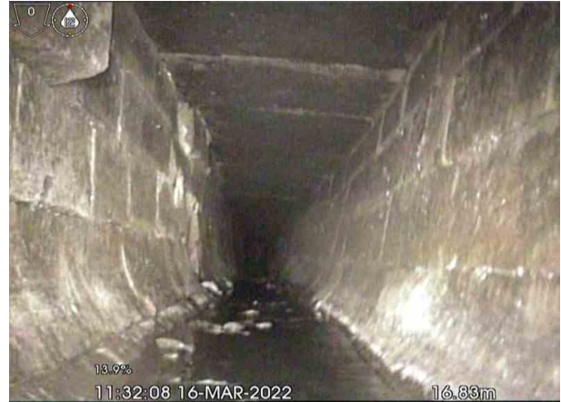
FW1X_e6eae0cb-a708-4923-b384-21f7473d81db_20220325_113926_689.jpg, 00:05:20, 16.83 m Settled deposits, fine, 10% cross-sectional area loss
