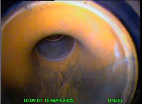
Upstream AX_05fba197-0138-4ba2-8a5e-4def130e685b_20220325_110 008_194.jpg, 00:00:06, 0.03 m Open joint, medium
