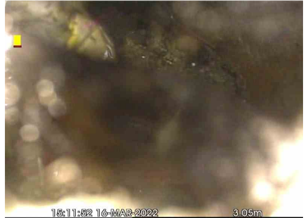
15:11:52 16-MAR-2022 3.05m G4X_85d306e3-1930-4205-adca-cf8b8c4505d7_20220328_111723_938.jpg, 00:00:17, 3.05 m Collapsed drain or sewer
