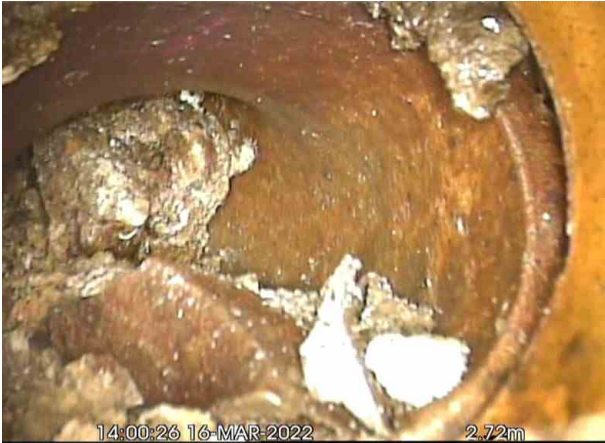
Upstream DX_69da25b6-9ce7-4ede-9e5f-d45e484d3679_20220328_09 4624_431.jpg, 00:00:14, 2.72 m General remark, Not in use
