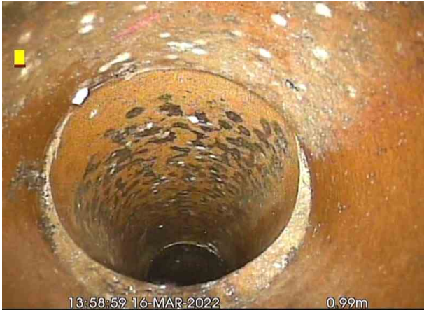
Upstream CX_d54a2afe-a992-4310-b46b-aa03cded51ee_20220328_09 4322_567.jpg, 00:00:09, 0.99 m Joint displaced, medium
