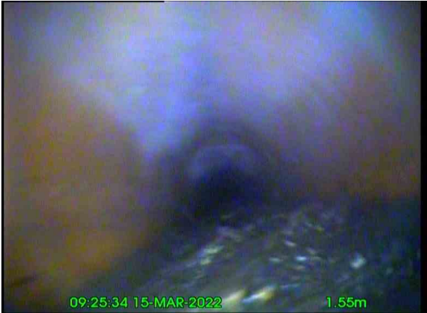
MH2X_6ed0165d-9cb4-4e35-bfa0-d64781de6bf2_20220325_095911_500.jpg, 00:00:18, 1.55 m Settled deposits, fine, 20% cross-sectional area loss, start
