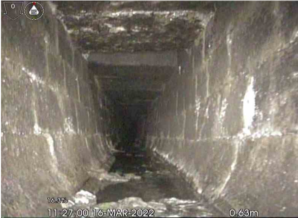
FW1X_a870c394-b1ae-4fb1-9286-213b03305d5b_20220325_113153_900.jpg, 00:00:13, 0.63 m Settled deposits, fine, 10% cross-sectional area loss, start
