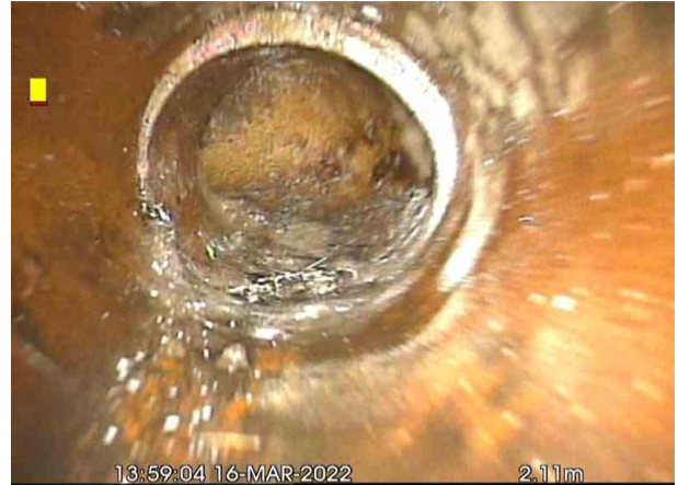
Upstream CX_9d66b288-b33d-4a4e-9219-ed65493c2be2_20220328_09 4356_650.jpg, 00:00:14, 2.11 m Joint displaced, medium
