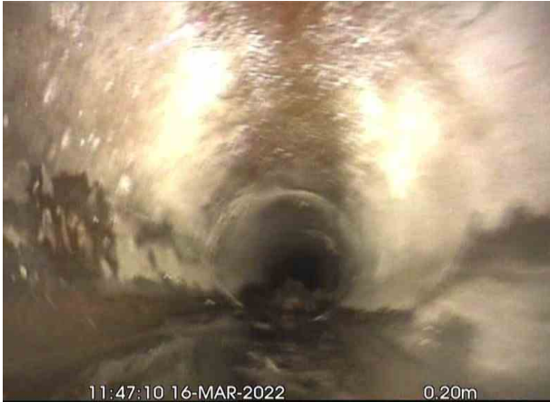
Upstream AX_2c24e93e-4de1-43ce-b970-b5e972d89093_20220325_144410_439.jpg, 00:00:06, 0.20 m Settled deposits, fine, 10% cross-sectional area loss, start
