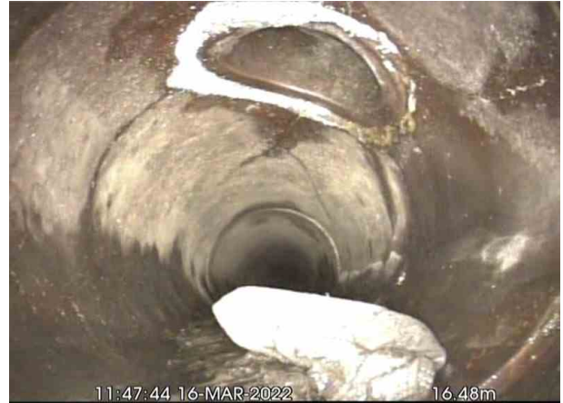
Upstream AX_8812d512-7283-4989-b0ff-8ae268397e0a_20220325_144603_711.jpg, 00:00:37, 17.06 m Settled deposits, hard or compacted, 20% cross-sectional area loss
